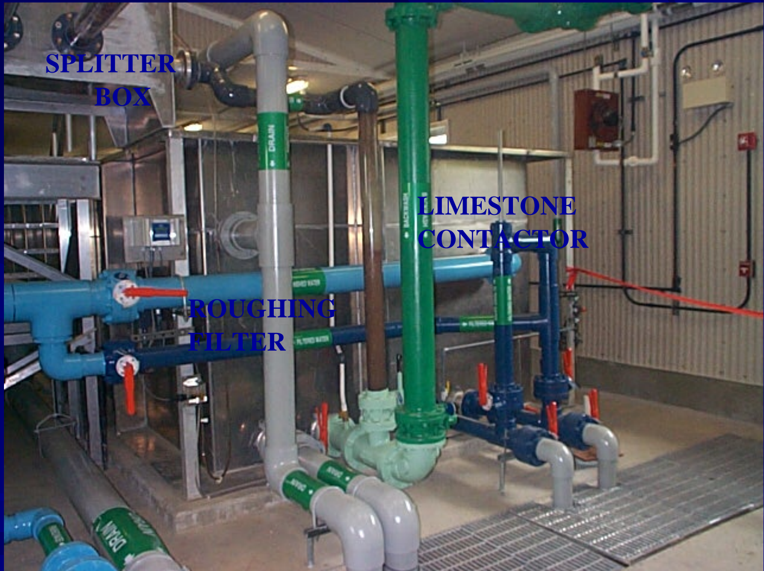
NORTH HAVEN, ME FILTER PIPE GALLERY
