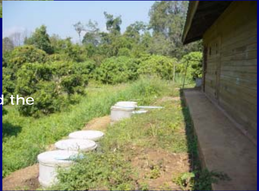
Gray water pipes disposing behind the boys' toilets
