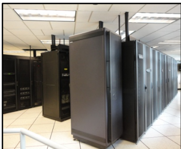
2,000 sq.ft. Lenharth Data Center: Recently renovated with a new energy efficient design.
