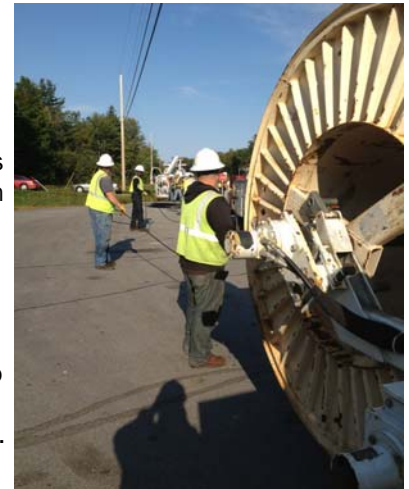
New Hampshire Optical Systems' contractor Waveguide has constructed aerial fiber in Gorham, NH.
