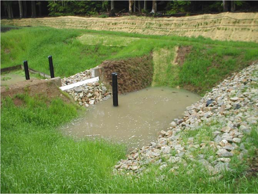
Flooded Sand Filter with Sedimentation Forebay
